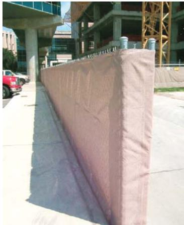
Perimeter fencing in accordance with TMC specifications
