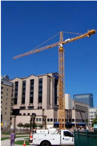
Cranes should be designed to withstand wind forces as required by federal, state and local codes and regulations
